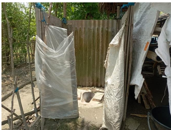
A rudimentary ring slab pit latrine toilet in rural Satkhira constructed with tin sheets, bamboo sticks, and plastic sheeting. Without a lockable door or roof, this structure offers minimal privacy and security. Location: Ashashuni, Satkhira, May 2025. © Amnesty International
